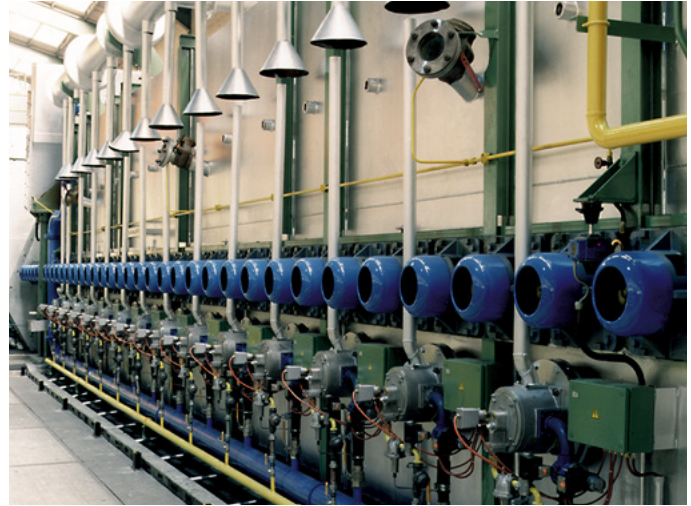
Roller hearth furnace
