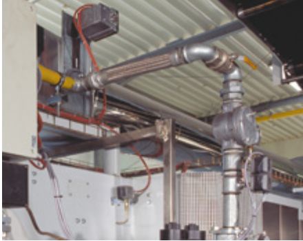
Stainless steel flexible tubes in the supply lines of buildings
