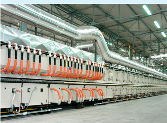
Roller hearth furnace
