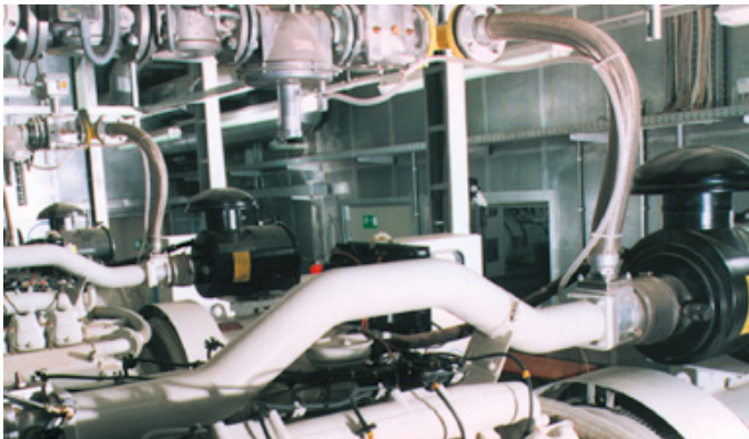
Gas engine in a combined heating and power plant
