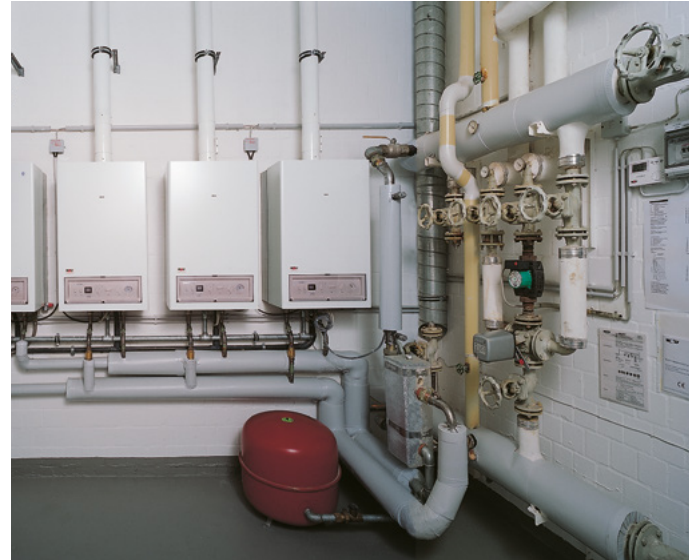
Heating boilers connected in cascade
